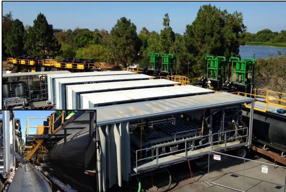
Sediment Dewatering Belt Presses
